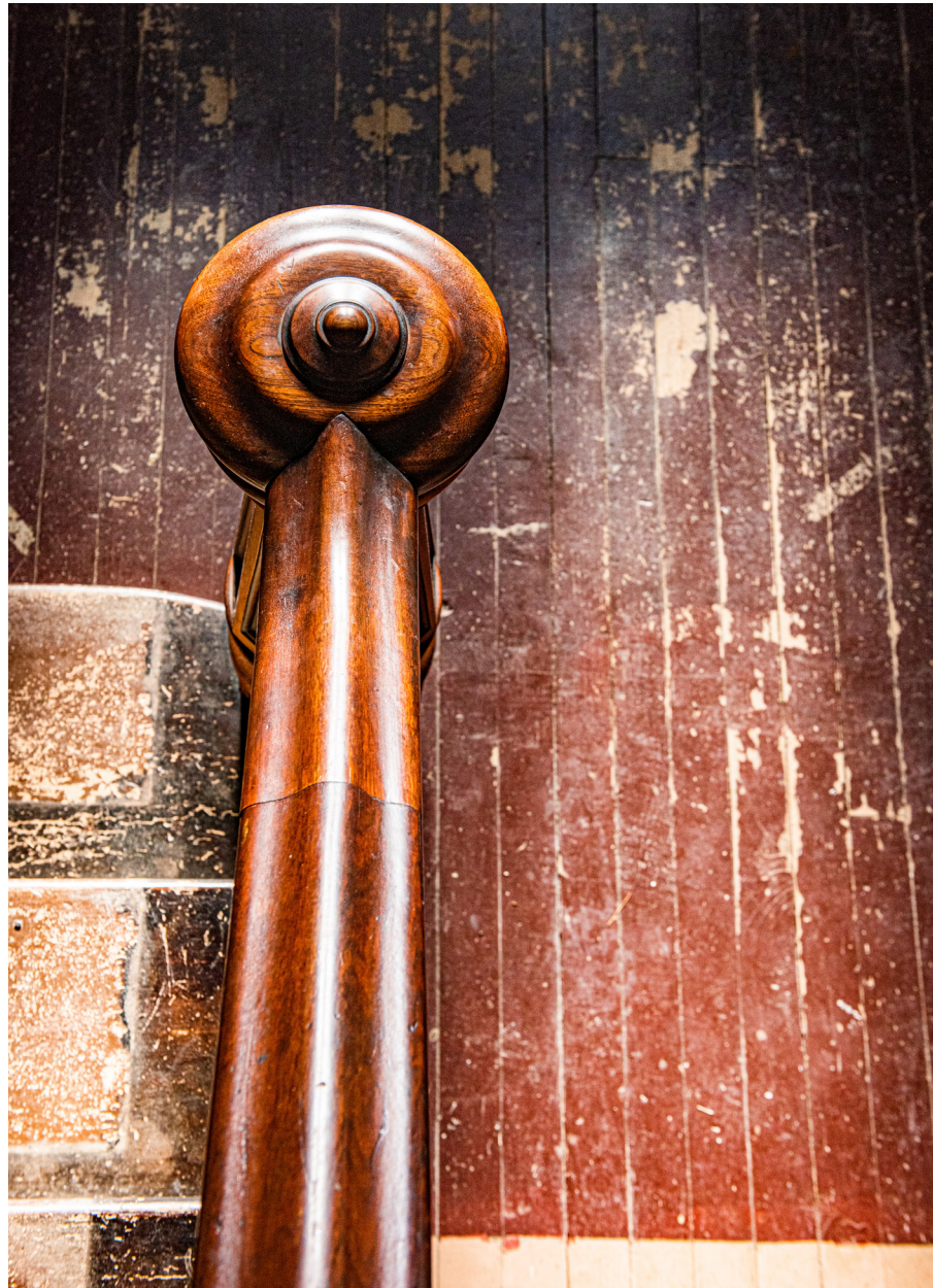
An overhead view of the carefully pieced newel post on the center-hall staircase in the Milanville home.
